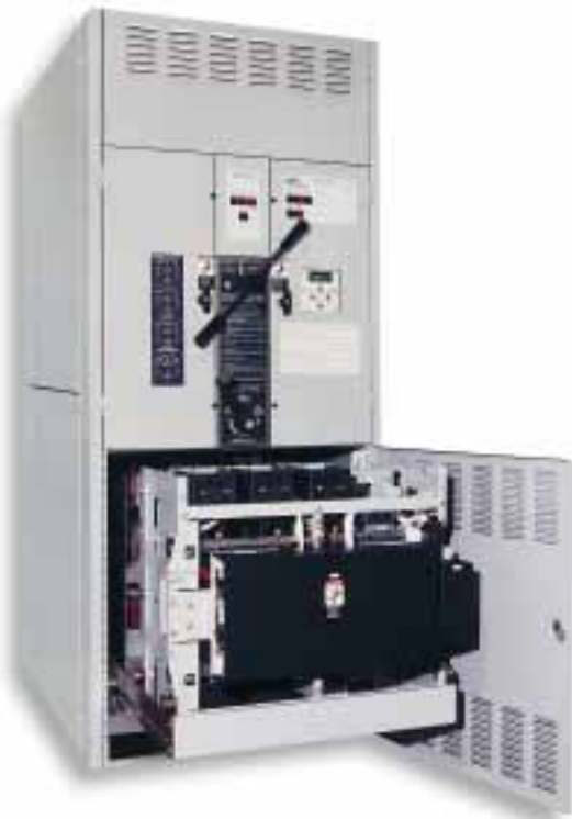
Fig. 5 Bypass-Isolation Transfer Switch rated 4 pole 2000 Amperes.
