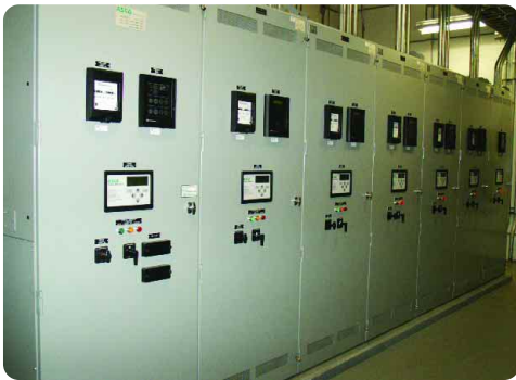
Above: The switchgear parallels the four generator sets, all of which and are interconnected to Pepco and the PJM Grid.
